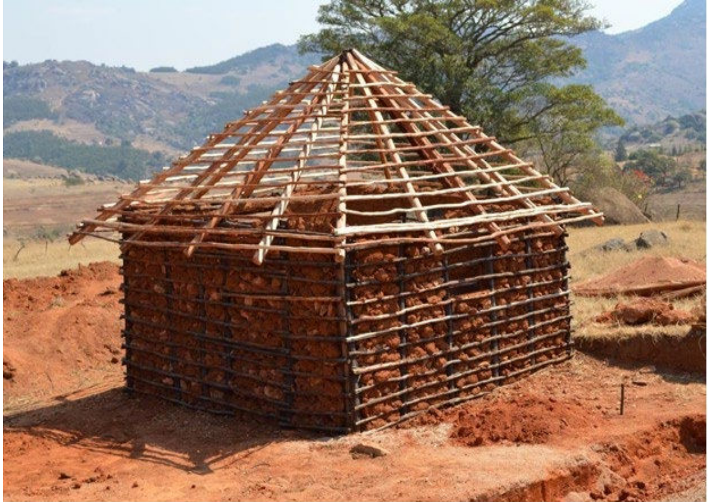
This home in Swaziland is constructed with wooden poles. The walls are filled with rocks, which will then be plastered over with mud. (Jon Sojkowski)
