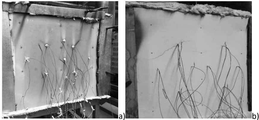
Fig. 8. a) Discolouration on the ambient side gypsum plasterboard; b) Discolouration and cracks on the ambient side magnesium sulphate board, after the fire tests
