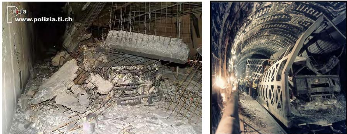
Fig. 1. a) Sectionally collapsed ceiling in the Gotthard Tunnel after the fire of October 24, 2001; b) Burnt out lorry transporter in the Channel Tunnel between the UK and France (fire incident on Nov. 18, 1996).
