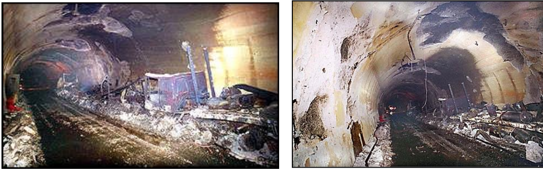
Fig. 6. The Mont Blanc Tunnel after the fire in 1999
