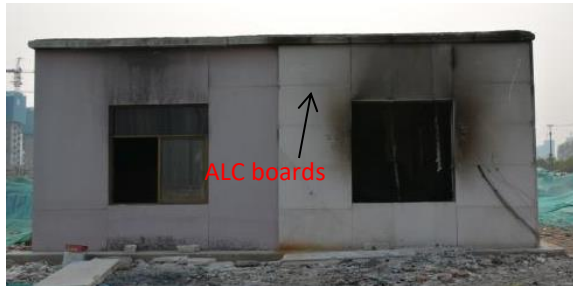
Fig. 19 Overall damage of the structure
