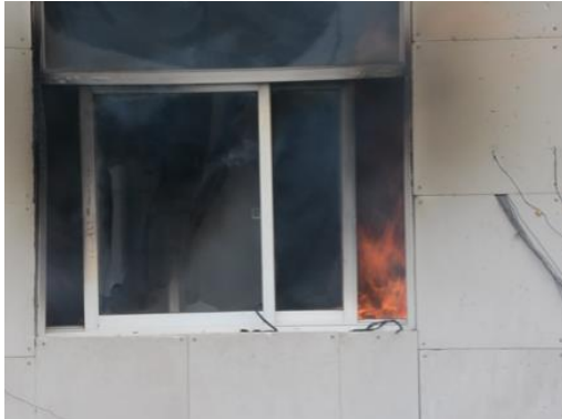
Fig. 15 Obvious cracking of window glass
