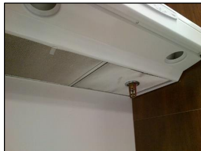
Figure 63 - Protectospray nozzle in hood
