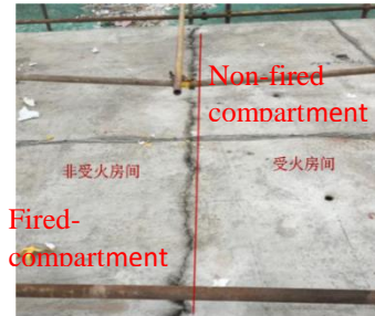
Fig.20 Crack on the concrete roof surface
