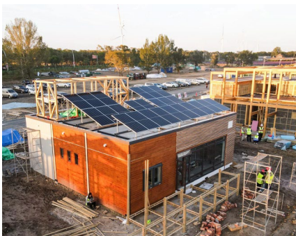
Figure 11. Photos of PVT module on the roof
