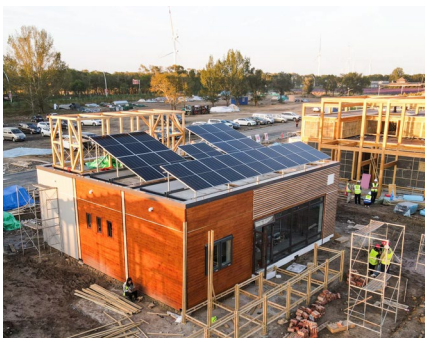
Figure 11. Photos of PVT module on the roof
