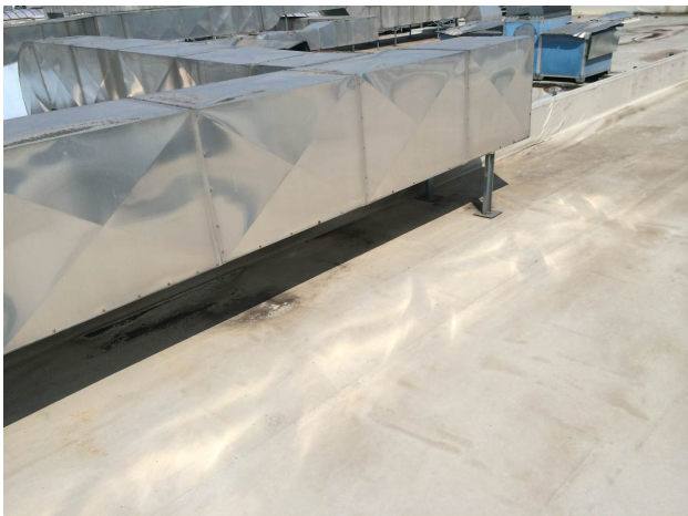
Figure 8: Solar reflection from metal duct onto TPO roof membrane
