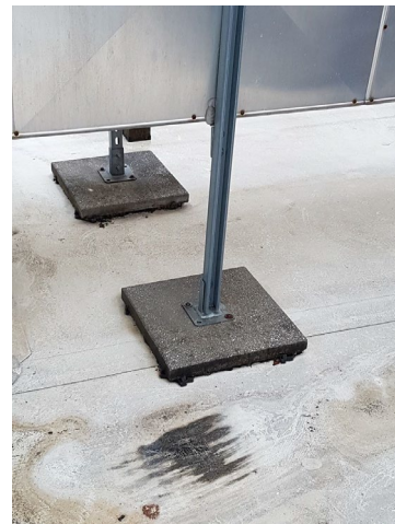
Figure 9: Local damage caused by concentrated heating
