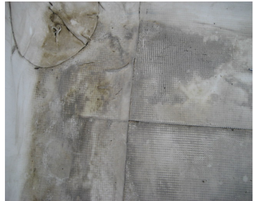
Figure 7: Isolated area of degradation
